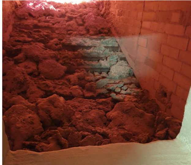
Fig. 3. Boiler moving grate surface during emergency stop
